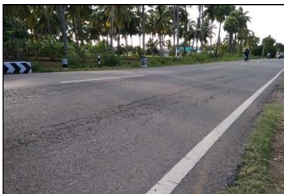
Alligator cracks at km 2/000 (SH 222)
