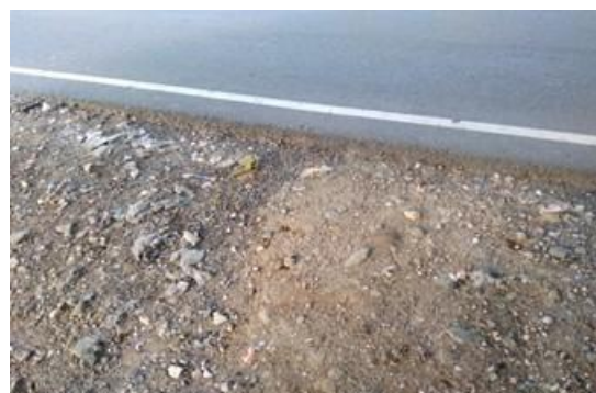
Edge drop at km 2/600
