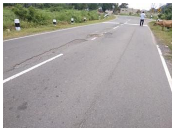
Potholes at km 86/550
