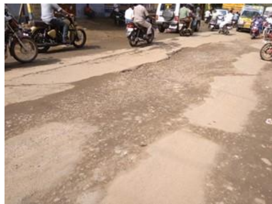
Distressed pavement at km 161/200
