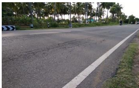
Alligator cracks at km 2/000
