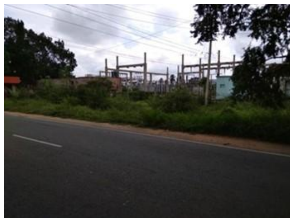
Substation RHS at km 89/180
