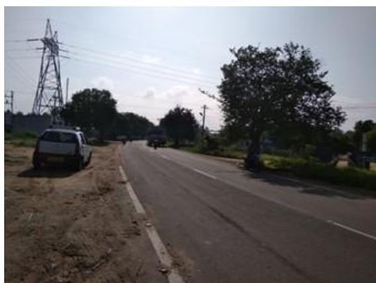
Longitudinal cracking at km 154/100
