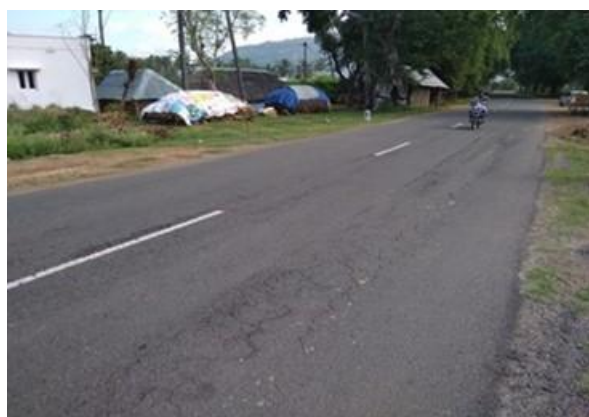
Alligator cracks at km 82/600
