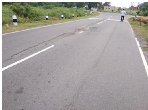
Potholes at km 86/550 (SH 30)
